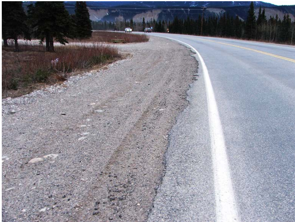
Healy Spur Road: Eroded shoulder
