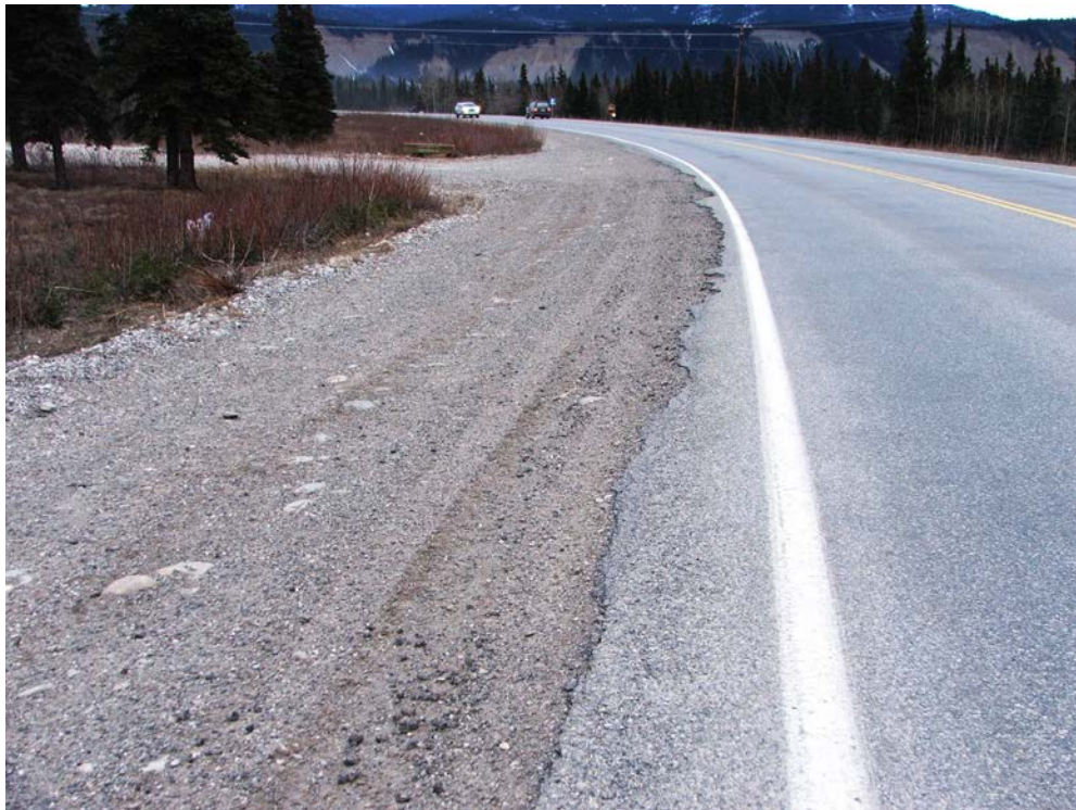
Healy Spur Road: Eroded shoulder
